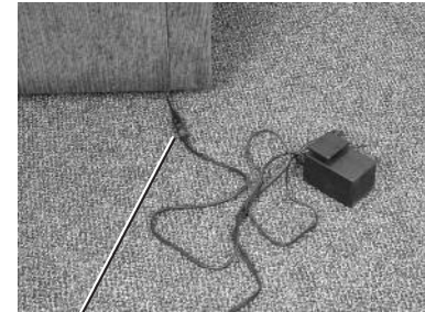
Power Transformer Connection
